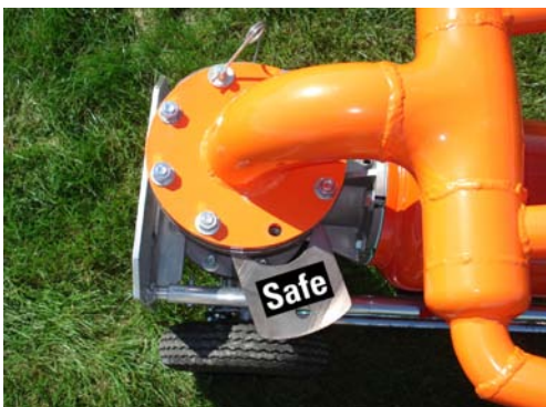
Position noted with “Safe” ticker.
